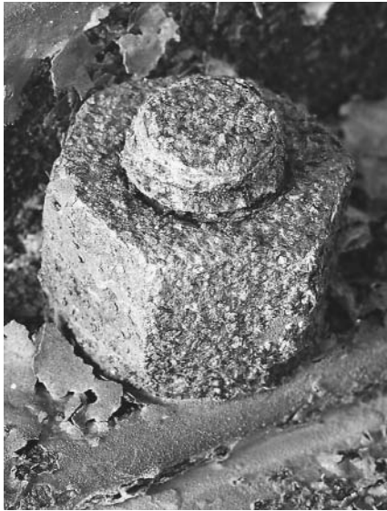
This metal bolt is rusted, a result of the oxidation of the iron metal of which it is composed.
