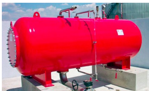
Figure 3-2. A tank of propane gas.
