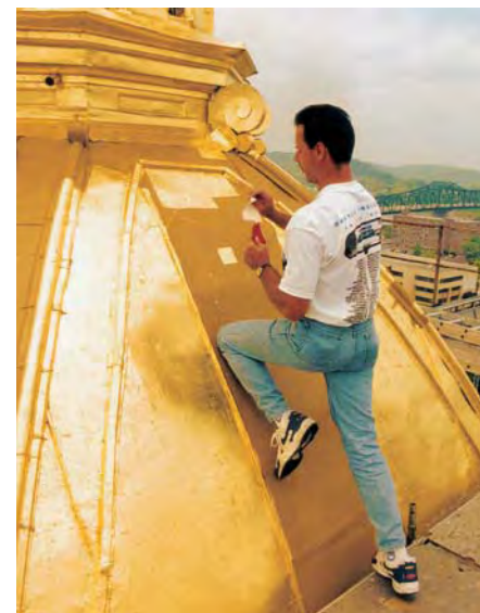
Gold leaf being applied to the dome of the courthouse in Huntington, West Virginia
