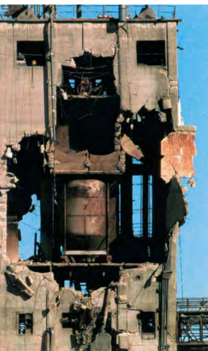
Figure 17.6 A grain elevator near Haysville, Kansas, was severely damaged by a grain dust explosion.
